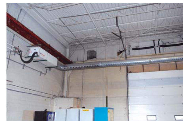
Extending the ductwork helped with slow recovery when an overhead door was opened.
