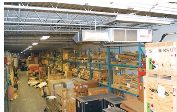
The heat pumps in the warehouse provide cooling as well as heating.
